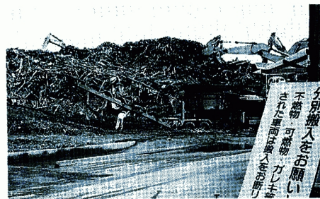
Photo 11 Chipping machine for wooden waste in the temporary storage location in Itami city.
