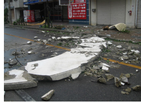
Photo 4 Fall down of wall
