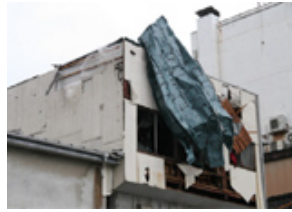
Photo 7 Hit by torn-off metal roof
