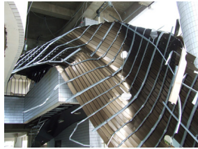
Photo 3 Fall down of ceiling panel
