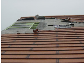
Photo 2 Torn-off roof tiles on gymnasium
