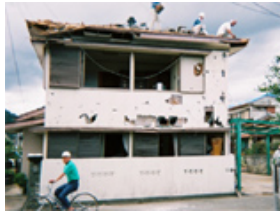
Photo 6 Damage by missile of tornado
