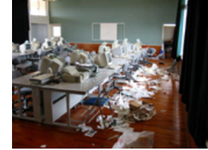
Photo 9 Interior damage by wind and rain
