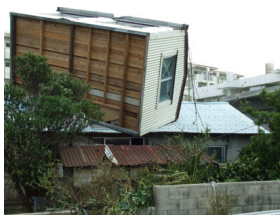
Photo 14 Lightweight prefabricated house got upon the neighbouring house
