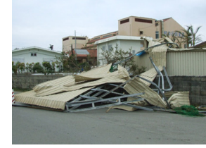
Photo 13 Collapsed partitioned sash with thick glass storehouse steel construction
