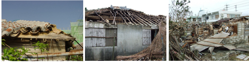
a. Tearing off of corner roof tiles b. Damaged roof c. Collapsed one
