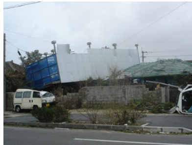
b. Lightweight steel storehouse got upon the neighbouring house.
