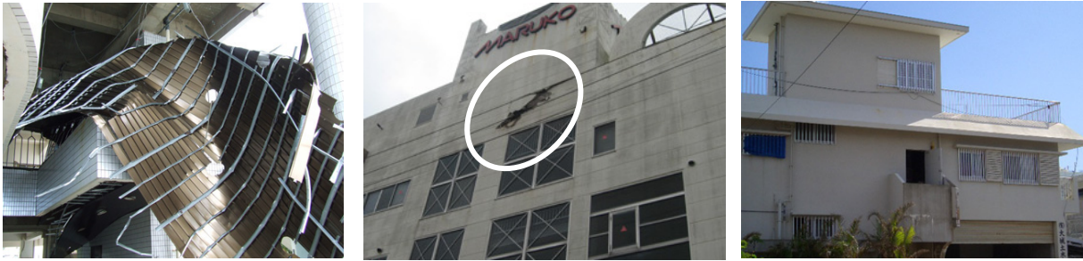
a. Fall down of ceiling panel. b. Damage to the wall. c. Protection with shutters and louvers.
