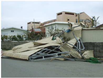
a. Lightweight steel storehouse collapsed.
