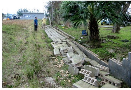
Photo 20 Fall down of block wall. (Ishigaki city office presents)
