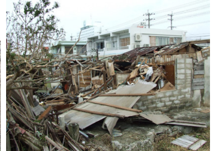
b. Completely collapsed house.
