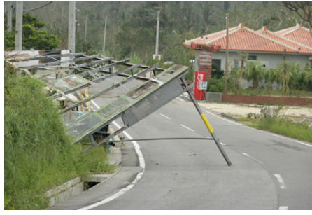
Photo 19 Fall down of fence. (Ishigaki city office presents)
