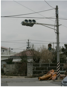
Photo 18 Distorted traffic signal. (Ishigaki city office presents)
