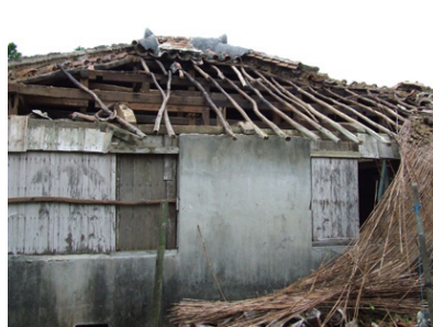
b. Blown off roof.
