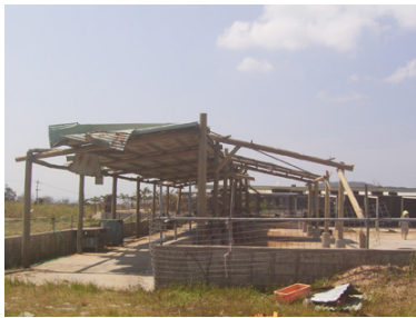
Photo 22 Blown-off of galvanized iron sheet from the cowshed.
