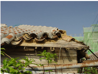
a. Damage to roof tiles.
