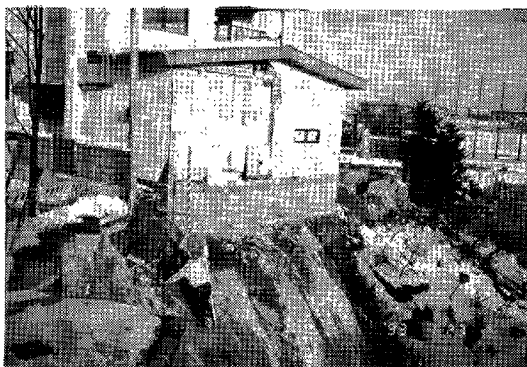
Photo 8 Damage of wooden house on the hill of Midorigaoka due to Kushiro-Oki Earthquake
