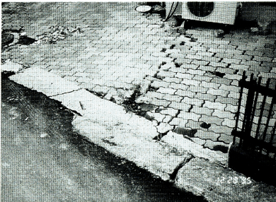
Photo.1 Cracks on brick floor and ground settlement in housing land
