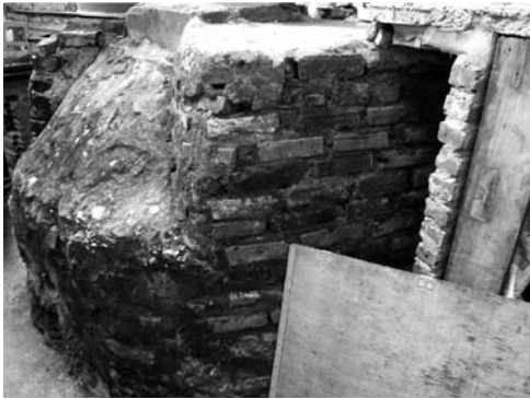
Fig. 18(c) Ruin of Wall at Position (9)
