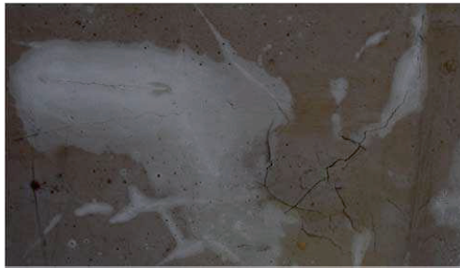
図4 Example of crack
