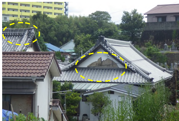
Photo 2 Damages of the roof and wall by windblast
