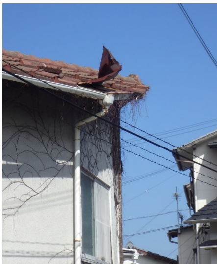
Photo 1 Damage of the roof by windblast
