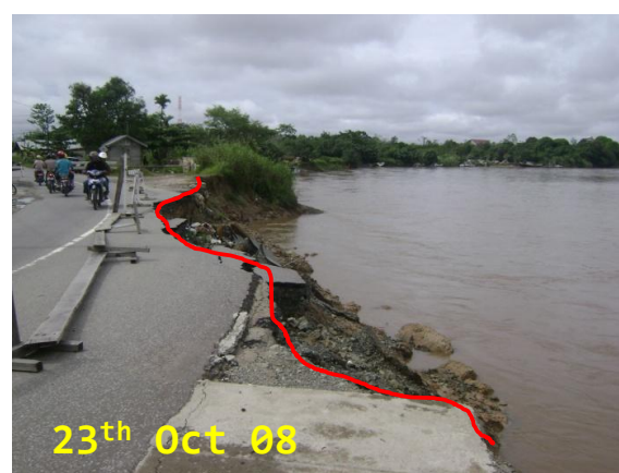
(b) Bank erosion
