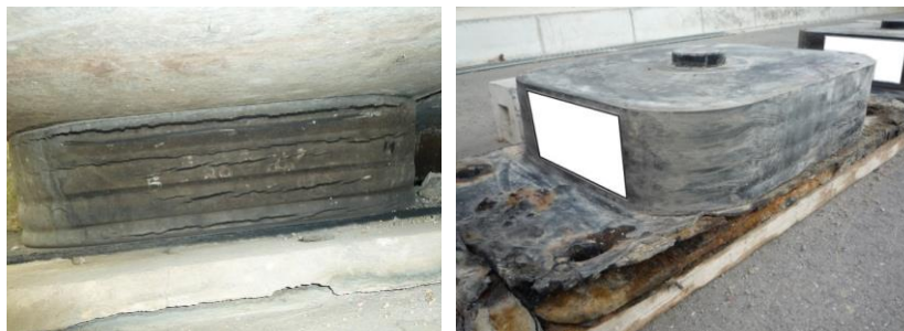
Figure 2.2 Damage status and cracks of ring bearings
