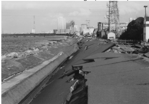
Fig. 1 Typical damage to river embankments (Yodo river embankment during 1995 Hyogoken Nambu earthquake) (after Ozutsumi et al, 2002)
