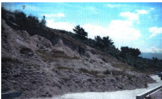
Fig.1 Picture of the slope failure
