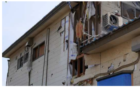
Photo 6 Damage to walls
