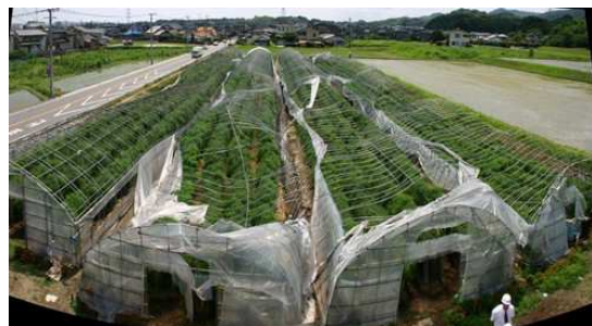
Photo 9 Damage to green house
