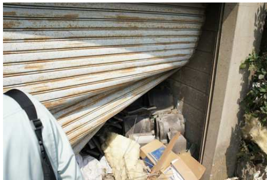
Photo 7 Damage to shutter
