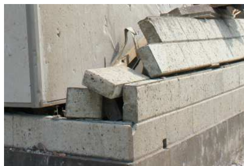
Photo 5 Damage to concrete-block wall
