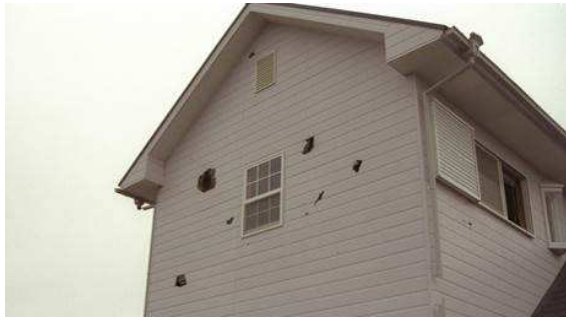
Photo 11 Damage by flying debris
