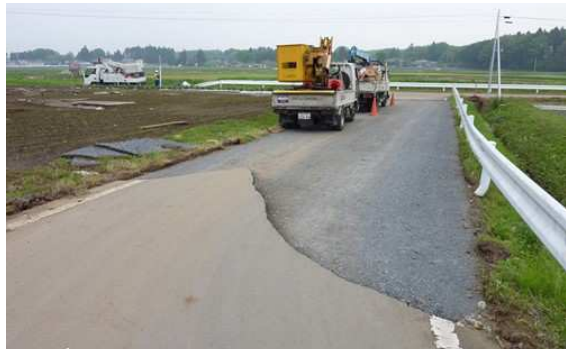
Photo 12 Damage to road surface
