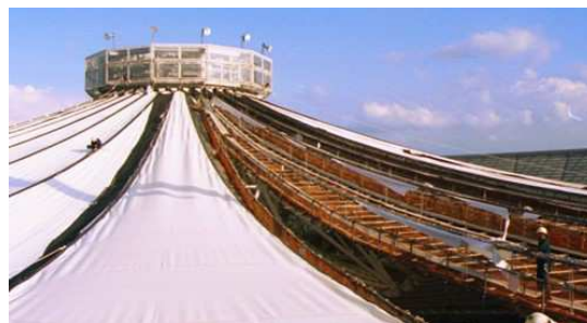
Photo 1 Damaged to membrane roof
