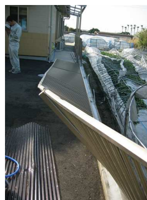
Photo 3 Damage to fence
