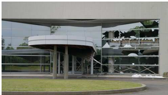
Photo 8 Damage to glass windows
