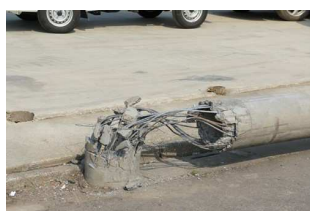
b, Electric distribution pole
