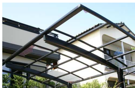
Photo 2 Damage to carport
