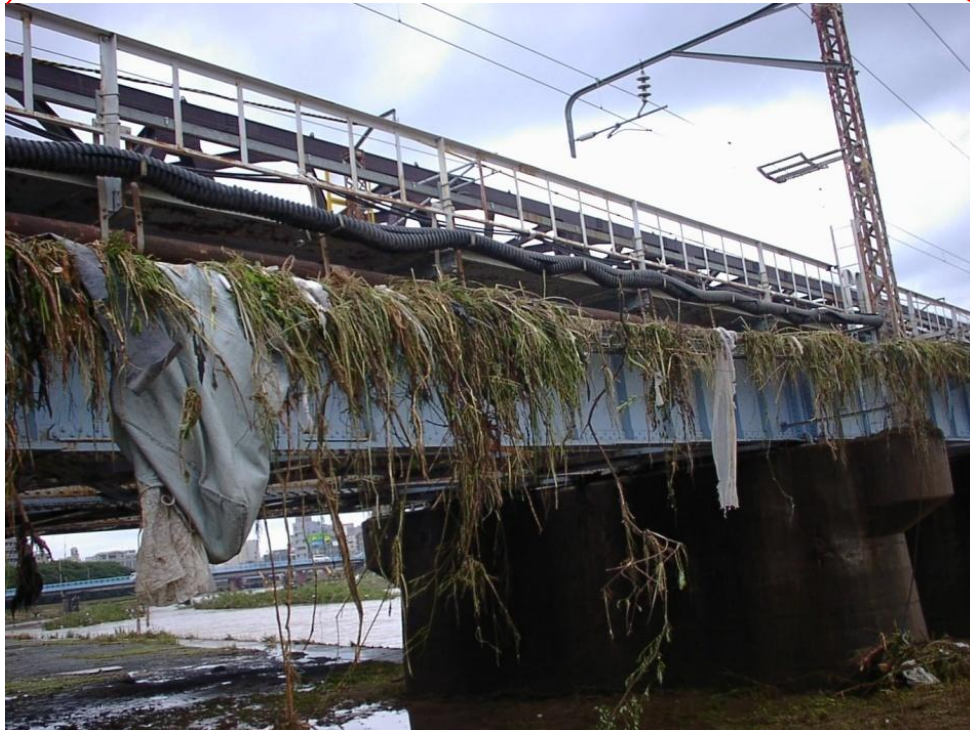
Figure 1.21 Water level rise (14cm) due to backwater by river structures in JR bridge (Photo Courtesy: MLIT, Japan)
