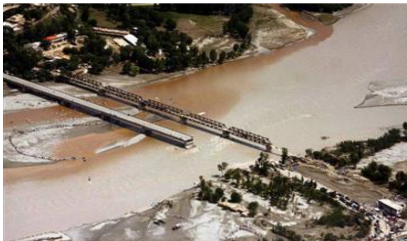
Figure 1.19 Bridge damaged by the flooding at Pakistan (Photo Courtesy: Pakistan National Disaster Management Authority)
