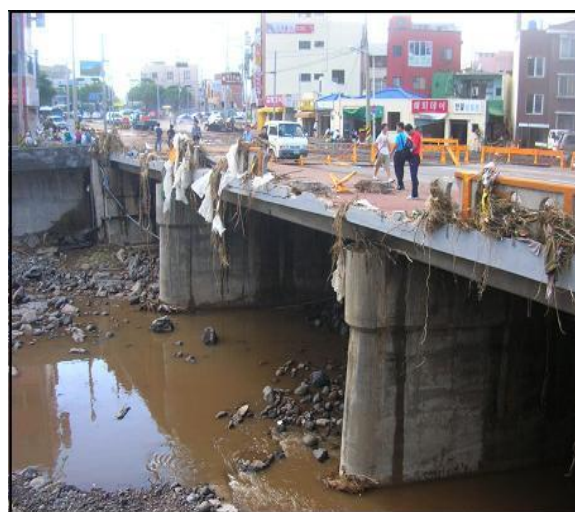
Figure 2 A bridge destroyed during Typhoon RUSA
