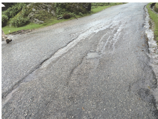
Figure 2 Puddles on a road in Bhutan
