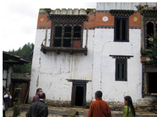
Photo 1b Damaged temple by 2011 earthquake in Haa (western Bhutan).
