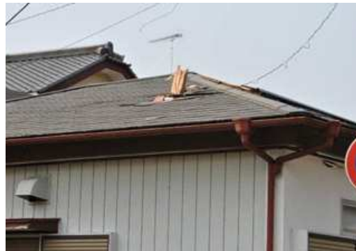
f. Timber stuck into a roof
