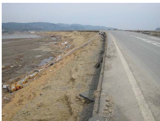
Figure 13 Washed embankment near the Shin Kitakami River
