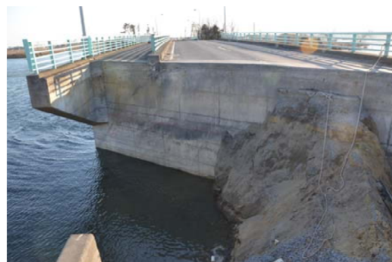
Figure 15 Lost embankment of Jokawa bridge.
