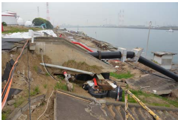
Figure 22 Damaged embankment in Kajima port
