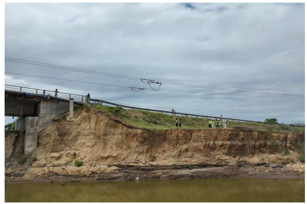
図-7-2 Sabaki Bridge橋台部の洗掘
