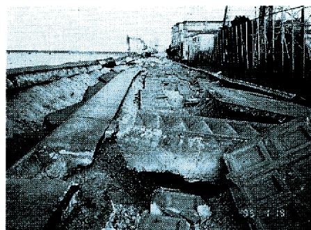
Photo 2 Perfectly collapsed embankment of Yodo River
