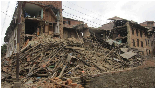
Building collapse near De-pukhu
