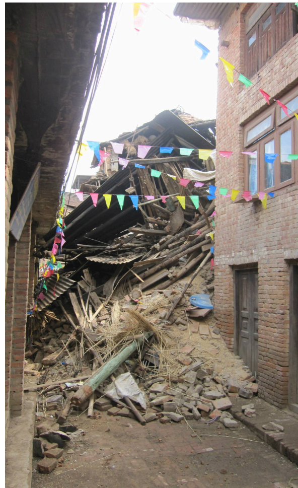
Blocked street in Bungamati
