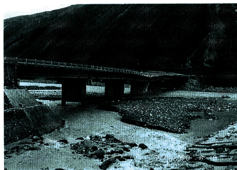
Photo 26 Damage to Dupinga bridge.
