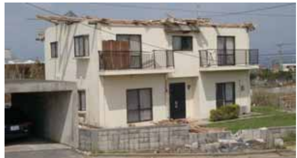
Photo 2 Badly damaged RC house ( courtesy Hirara city office )
