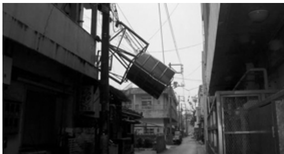
Photo 11 Fall of water tank (courtesy Hirara Tsutomu)
