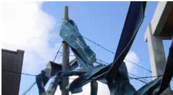
Photo 30 Roofing metal sheets twisted on electric pole ( courtesy Prefecture branch office )
