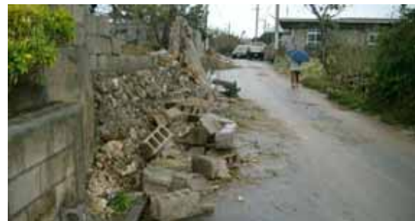
Photo 12 Fall down of concrete block wall (courtesy Miyakojima local weather station)
