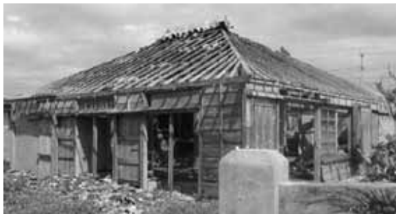
Photo 1 Completely destroyed wooden house
