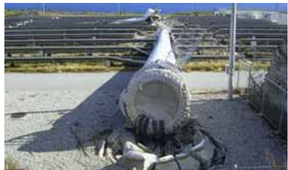
Photo 22 Broken down tower ( Okuda et.al. 2003 )
