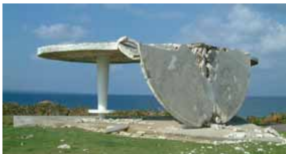
Photo 13 Damage of observation deck (courtesy Hirara city)
