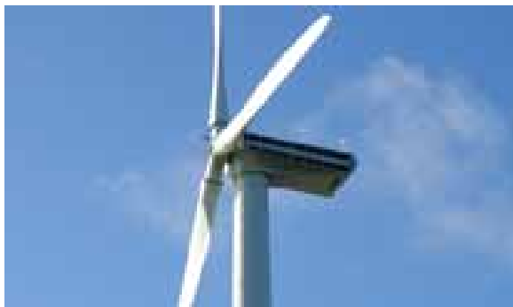
Photo 21 Nacelle cover was blown off ( courtesy Building Research Institute )
