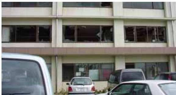
Photo 3 Damage of openings (courtesy Okinawa Prefecture )
