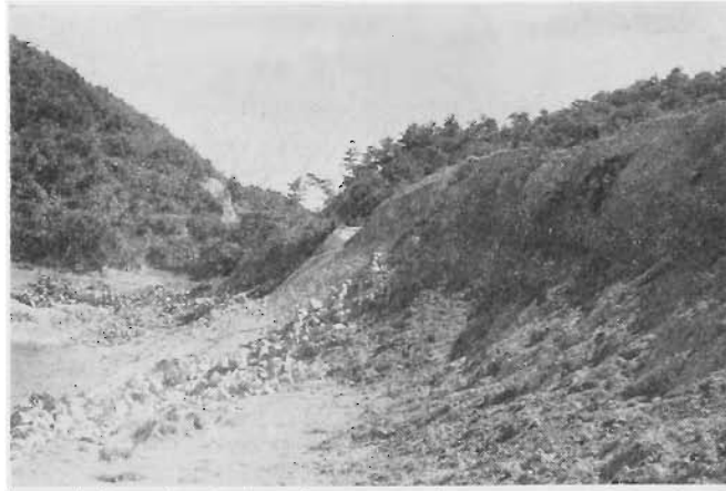
Photo. 7 Secondary failure of upstream slope due to rapid-drawdown.
