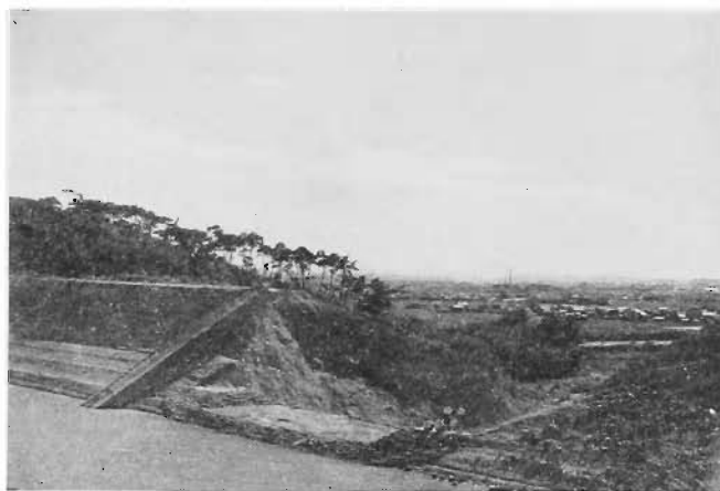
Photo. 6 Primary failure of downstream slope due to full reservoir.
