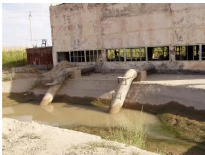
Fig. 9 Water pumping station at Kumsangir (partly functioning)
