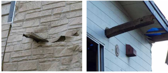
Fig. 1 Damage to the walls of houses by flying debris
