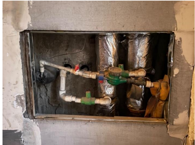
b) The doors for the newly replaced water meter boxes have not been installed.
