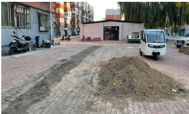
c) Some road surfaces have not been fully restored.
