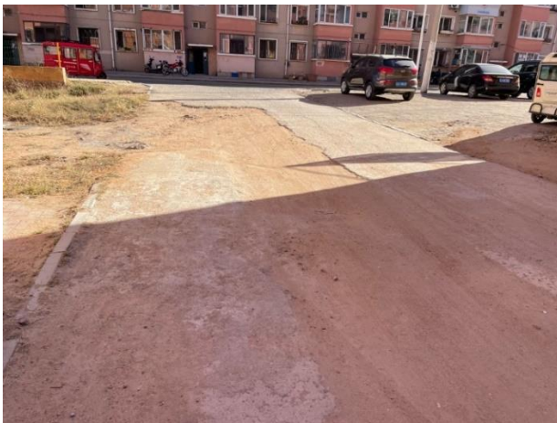
a) Some road surfaces have not been fully restored.
