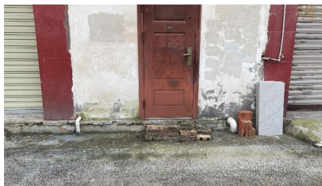
b) Frequently flooded road surface
