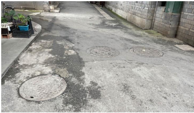
a) Damaged road surfaces
