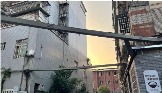
c) Overhead wires with protective sleeves
