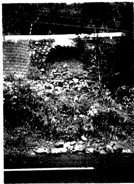
Photo 3 Damage of the edge of road
