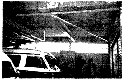
Photo 8 Buckling of horizontal braces
