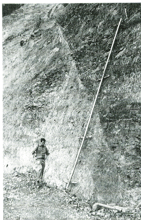
Photo 2. Northern part of the cut slope. A remarkable fault crosses the slope at the middle point of a pipe for an extensometer.
