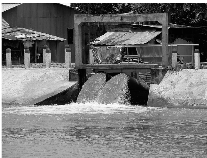
Fig. 7. Drain Pump Fixed at the Full-dike
