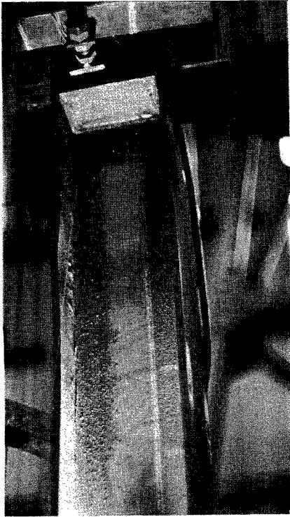
Photo. 8 Local buckling of column top (BC5).
