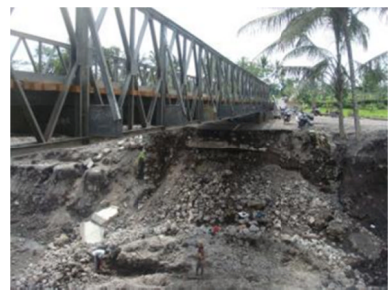
(c) Broken bridge in the middle reach of Opak River
