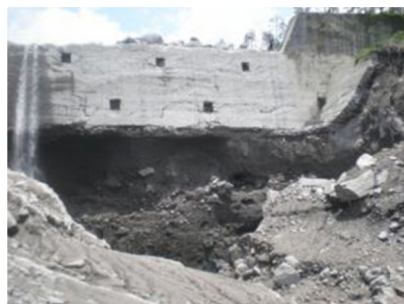
Photo 9(b) Collapse type 2
