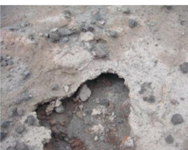
(b) Collapsed crust
