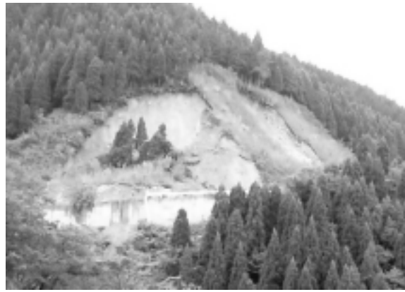
Photo 9 Collapse in road cut slope A
