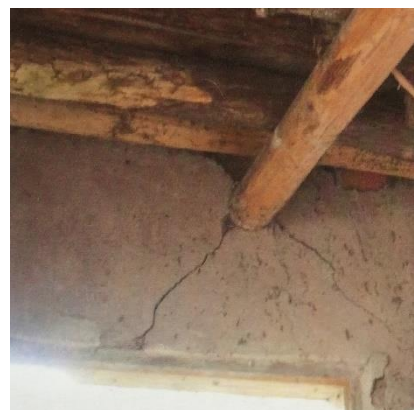
(b) Cracked backwall
