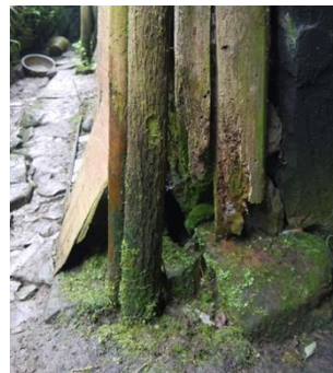
(f) Rotten pillars on spot (f)
