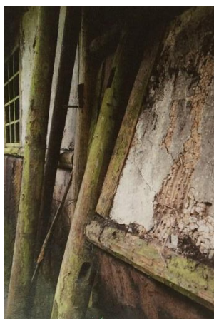
(c) Distorted wall and pillars
