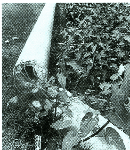
Photo 3. Broken electric line pole.
