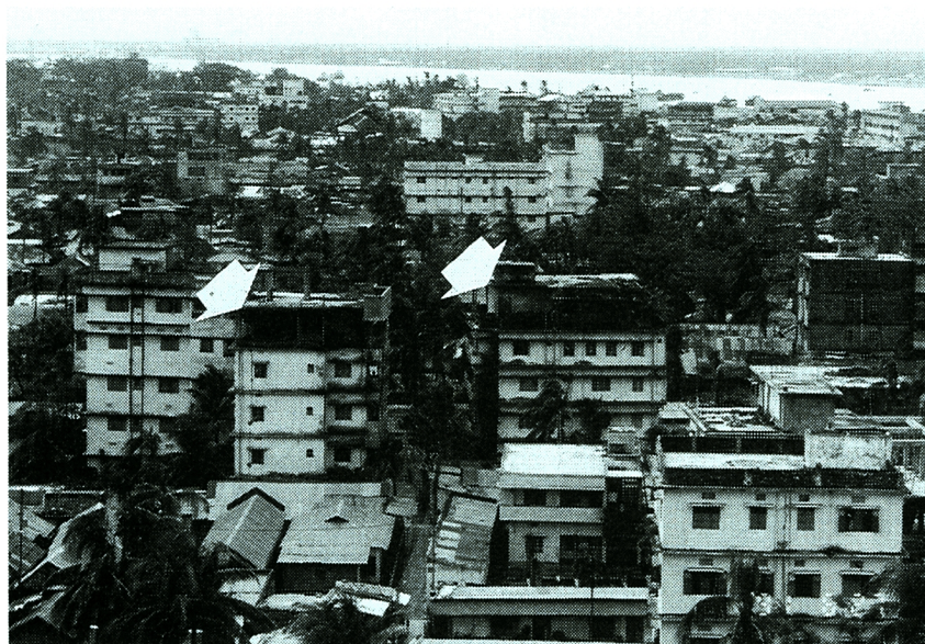
Photo 2. Blowdown brick walls.
