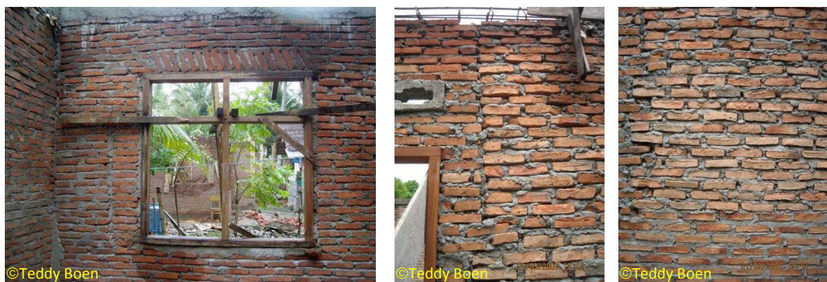
Figure 102 – Poor Workmanship Non-uniformities in Actual Brick Walls
