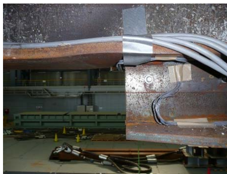
Figure 6.19 Fracture situation of connections (SL)
