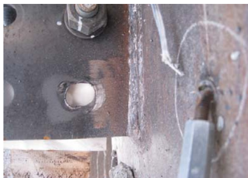
Figure 4.8 Deformation of bolt hole
