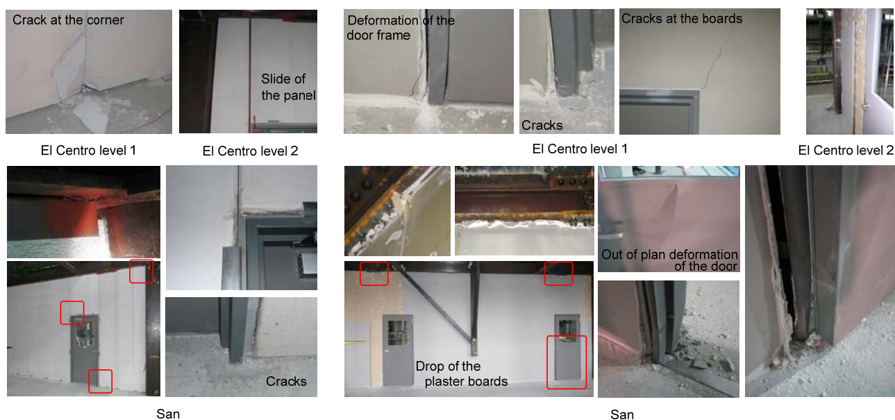
Figure 3.15 Damage to various nonstructural components
