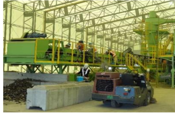
Figure 4-5: Separation, crushing and compression facilities
