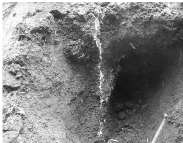
(b) Crack depth of 50 cm.
