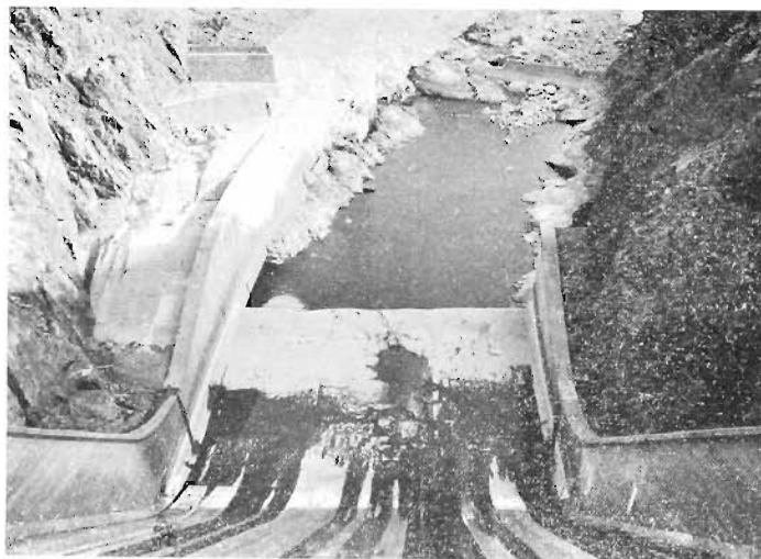
Fig. 15. Erosion at Nagayasuguchi Dam.
