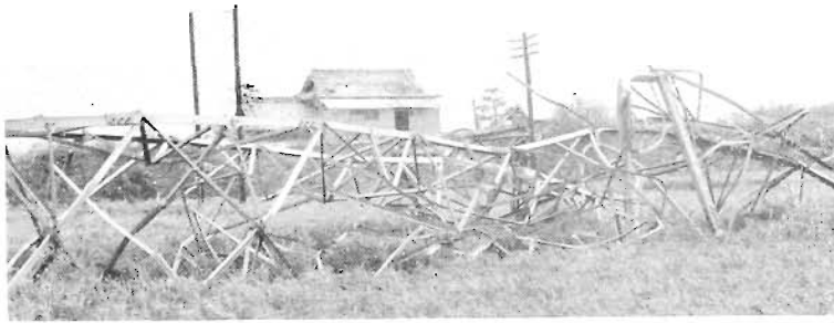
Fig. 1. Collapsed steel tower due to typhoon.
