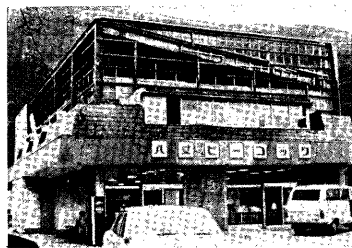
Photo. 12. Damage to external wall: steel frame.
