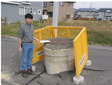
Fig. 1 Observed uplifted manhole after 2003 Tokachi-oki, Japan, earthquake.
