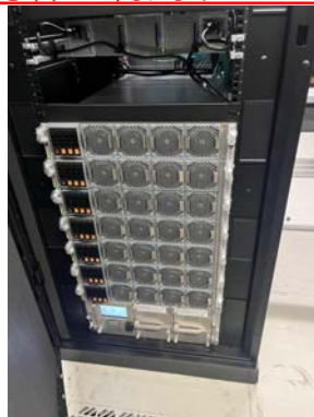
GPU nodes Installed in 2025.03
