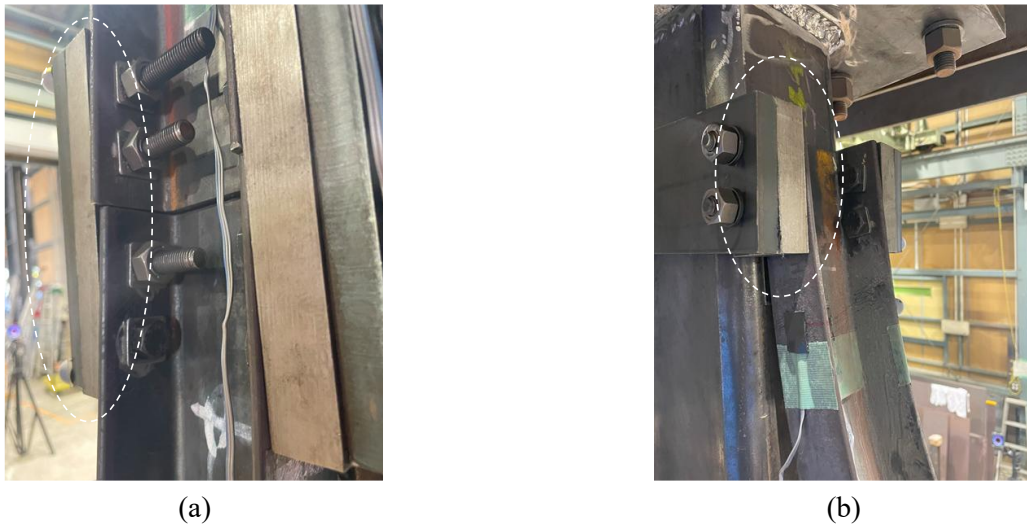
Figure 6-15 Photos of connection plate slipping at (a) middle and (b) top of the frame.
