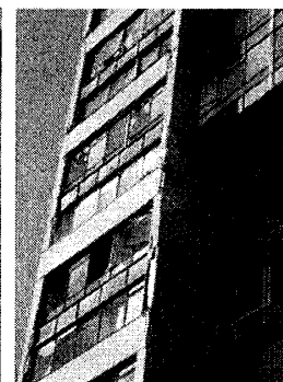
Photo 4 Damage of beam-wall joint
