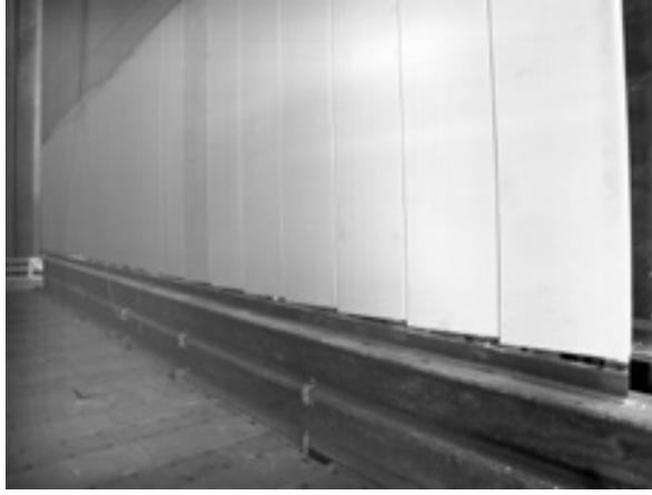
(a) Inclination of ALC Panels (1/25 rad Drift)
