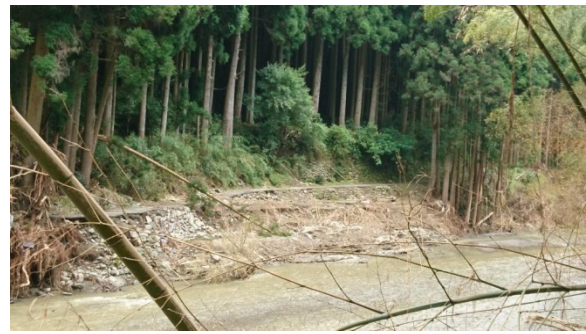
Photo 5 River bank erosion upstream of Terauchi Dam (Planted trees were discharged from the eroded bank)
