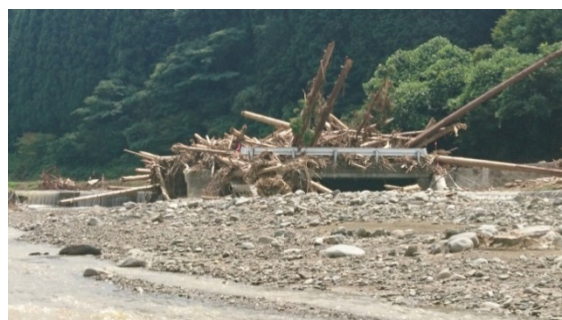
Photo 3 Bridge clogged by woody debris ( Kurokawa River upstream of Terauchi Dam )
