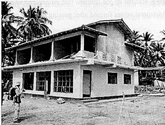
Photo 13 Barley damaged building made of concrete
